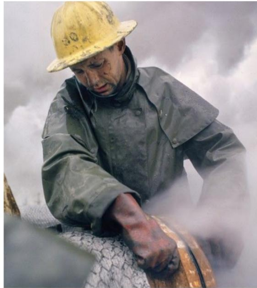
Maintenance engineer with protective clothing repairs a pipe connection that is leaking 221° Fahrenheit steam.
